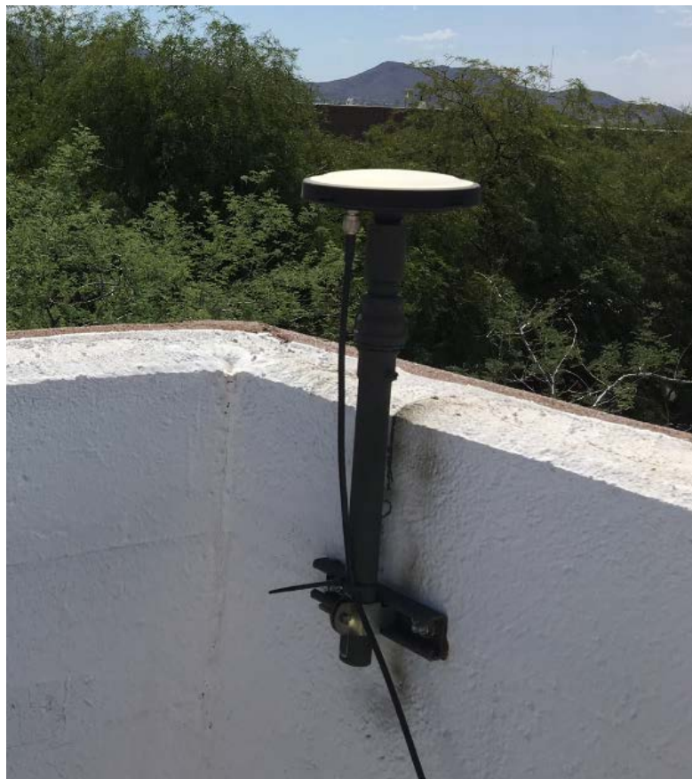
Figure 2-5: Roof mounted antenna
